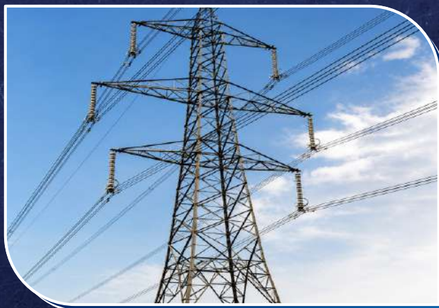
Transmission Line Towers
